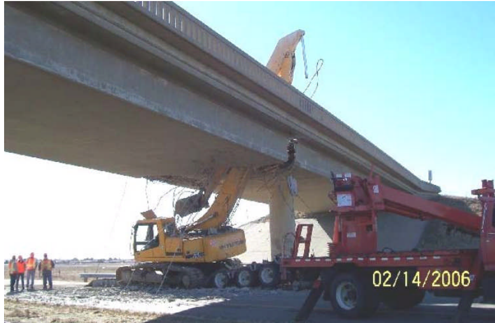
Figure 4.4.2 Accident Involving Construction Equipment and a Bridge
