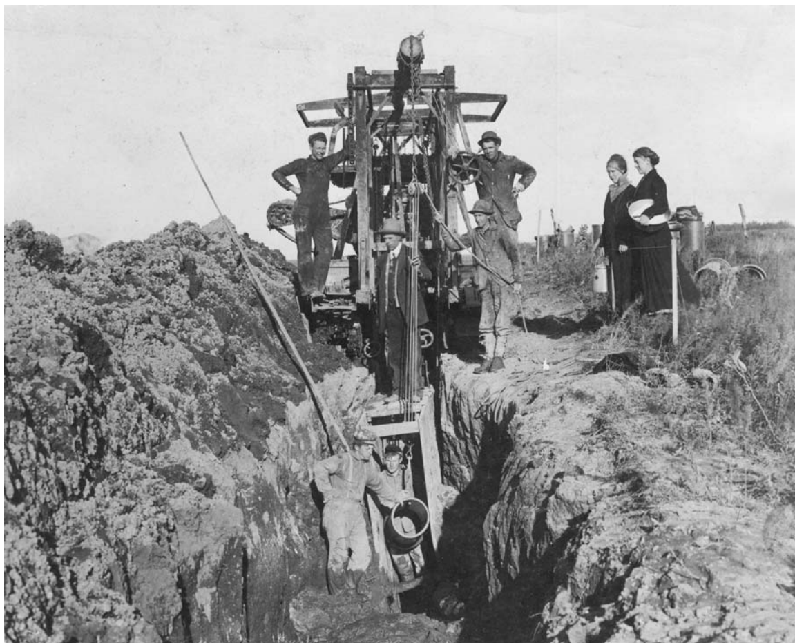
Laying subsurface drain tile with a machine. Shallow tiles and ditches were generally dug by hand. About four miles west of Dawson, Lac qui Parle County, circa 1905. (MHS photo)
