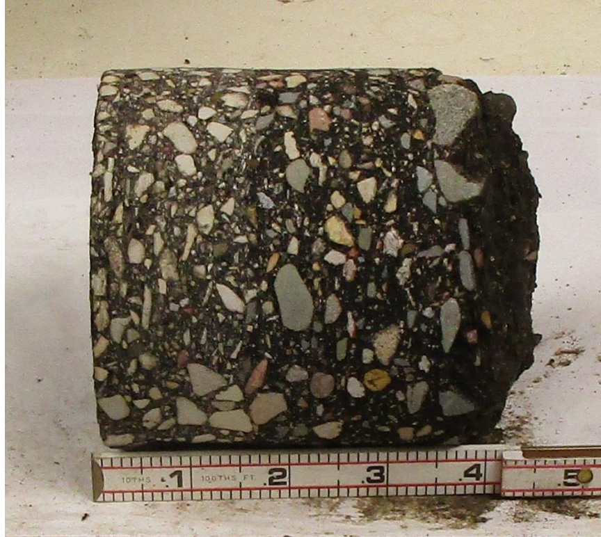
Figure 100.20 – Stripping of an asphalt core from the bottom of the asphalt layer.
