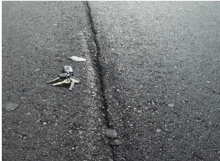
Figure 600.32 – Poorly compacted longitudinal joint
