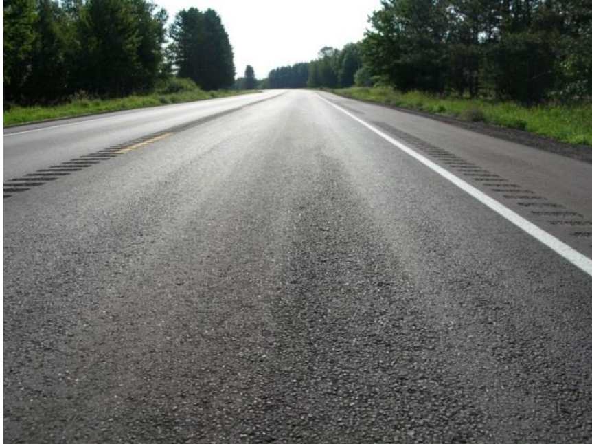
Figure 600.10 – Severely segregated pavement
