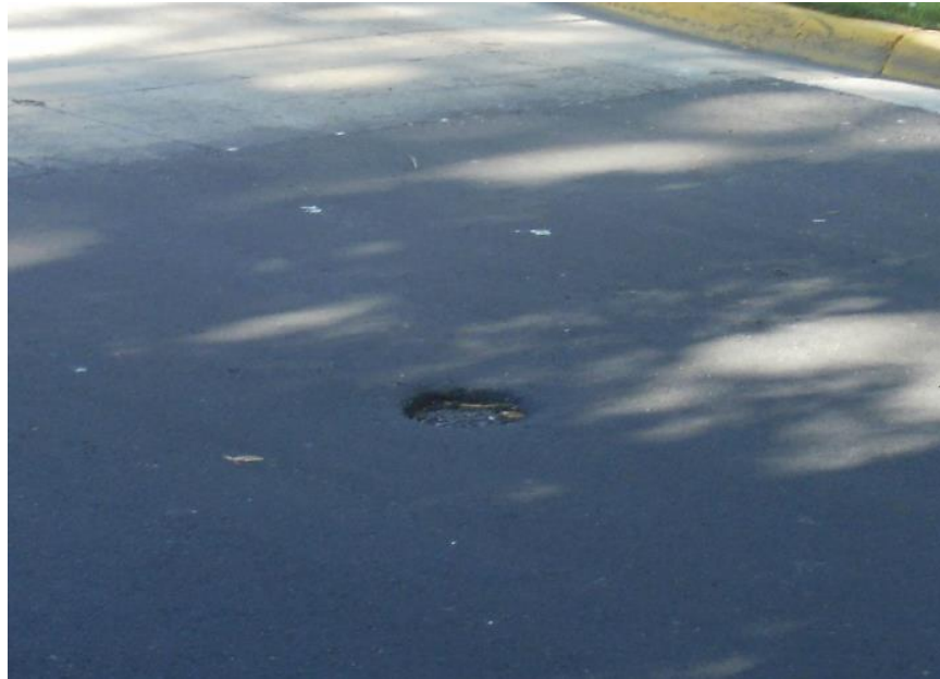
Figure 500.30 – Water valve box that has been adjusted too low.
