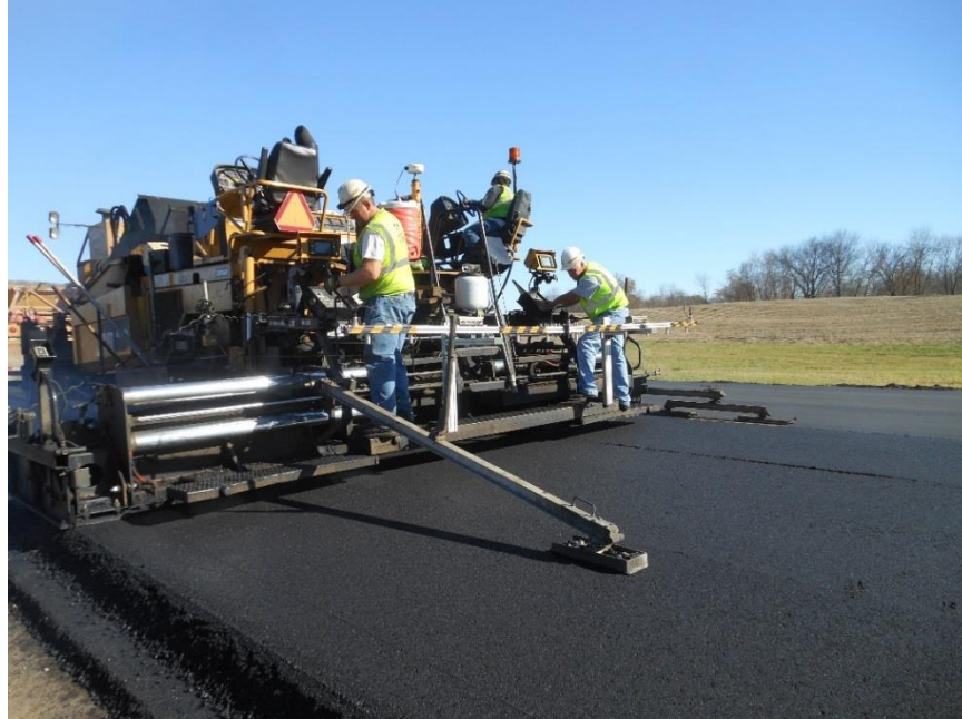
Figure 600.20 – Lines in the mat from incorrectly adjusted screed extensions.
