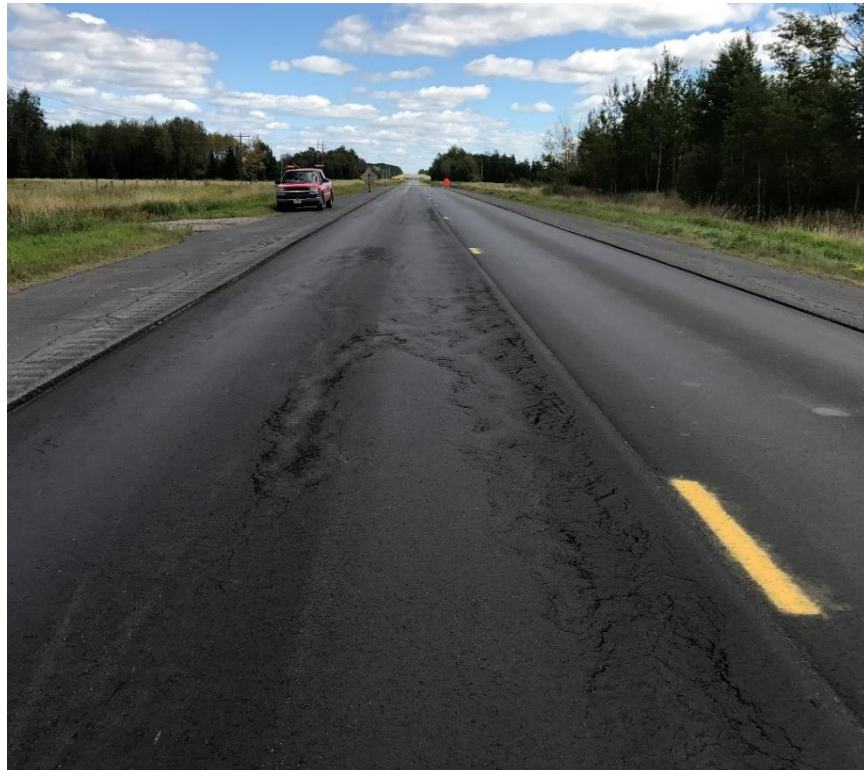
Figure 600.35 – This is what the road can look like the day after paving in the rain. All of the distressed areas shown will need to be removed and replaced.
