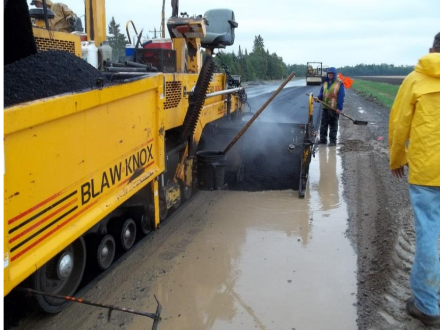
Figure 600.34 – Paving in the rain. When the paver creates a wake through the water, it is well past time to halt production. The situation pictured above should never be allowed to occur.
