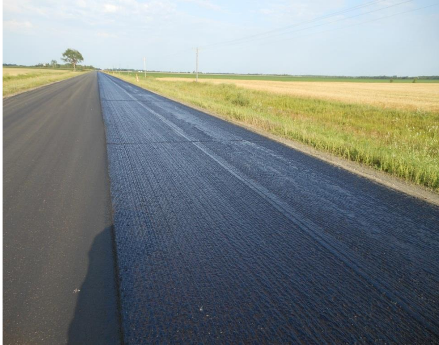
Figure 100.6 – Bituminous tack coat being used to bond an asphalt overlay to the milled surface of an existing bituminous pavement.
