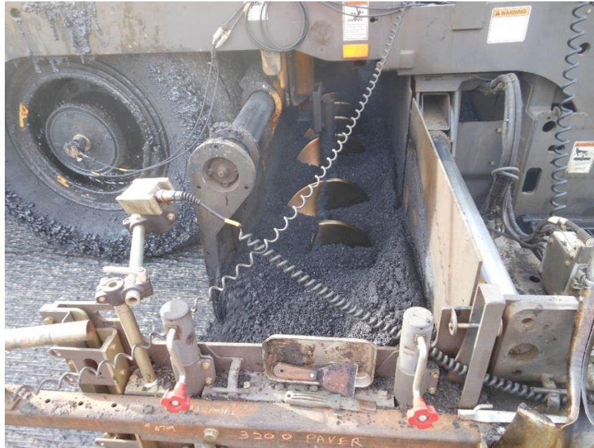
Figure 600.19 – This photo shows the correct material head in front of the screed. However, auger extensions should have been used in this case.
