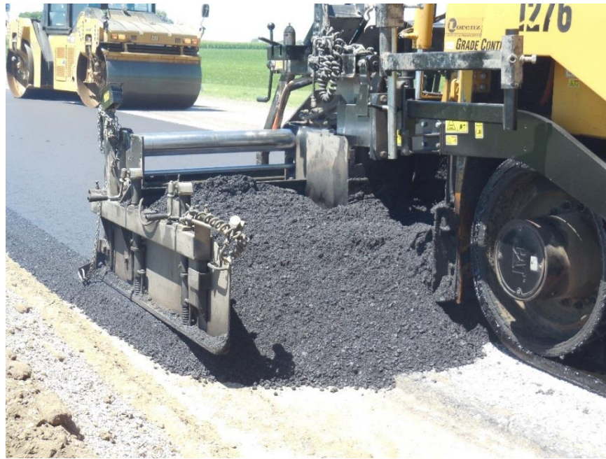
Figure 600.18 – Excessive material head in front of the screed. The augers should not be buried.
