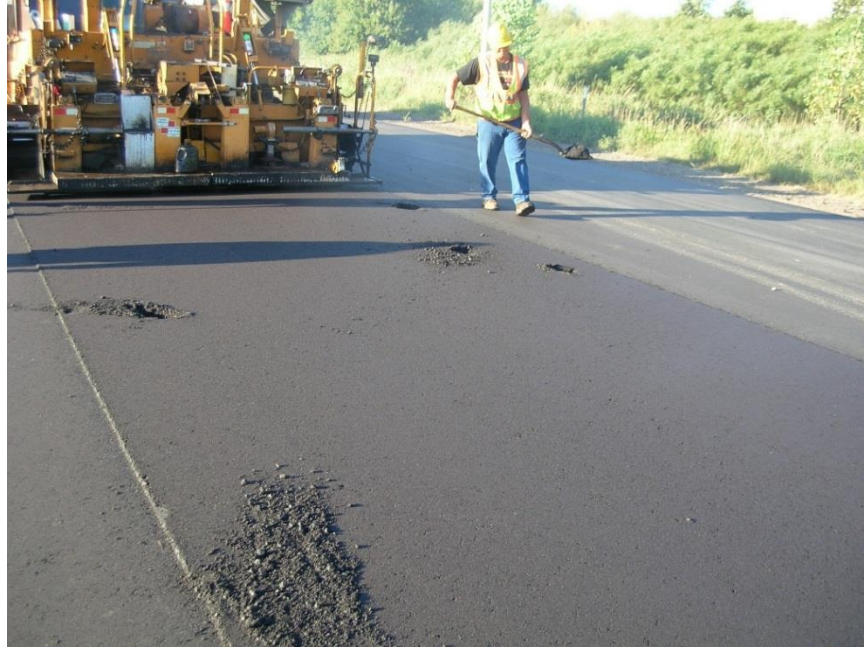
Figure 600.38 – Removal of cold chunks from the bituminous mat. The areas will have to be filled in by hand, and will likely be areas of localized segregation. Paving operations should halt if this continues.
