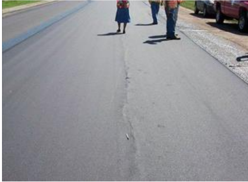
Figure 600.14 – Blistering of the mat in the tender zone
