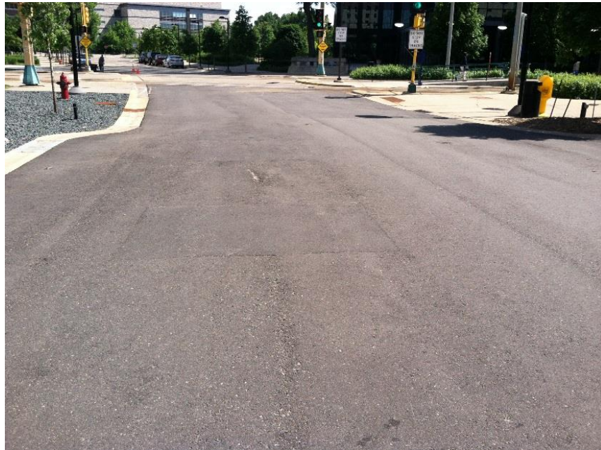
Figure 100.14 – Bituminous patch over raveled pavement.
