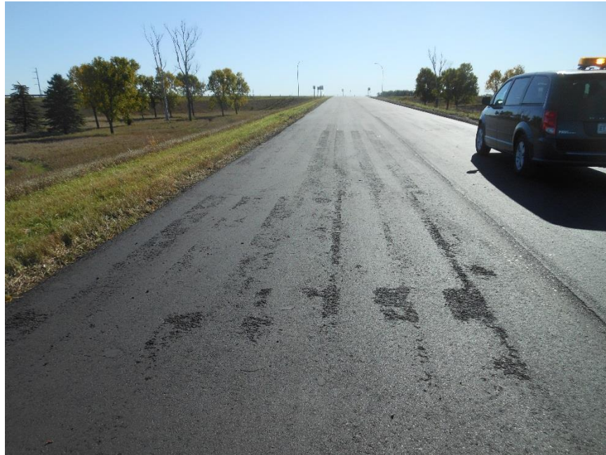
Figure 500.32 – Unacceptable mixture pickup from pneumatic tired roller
