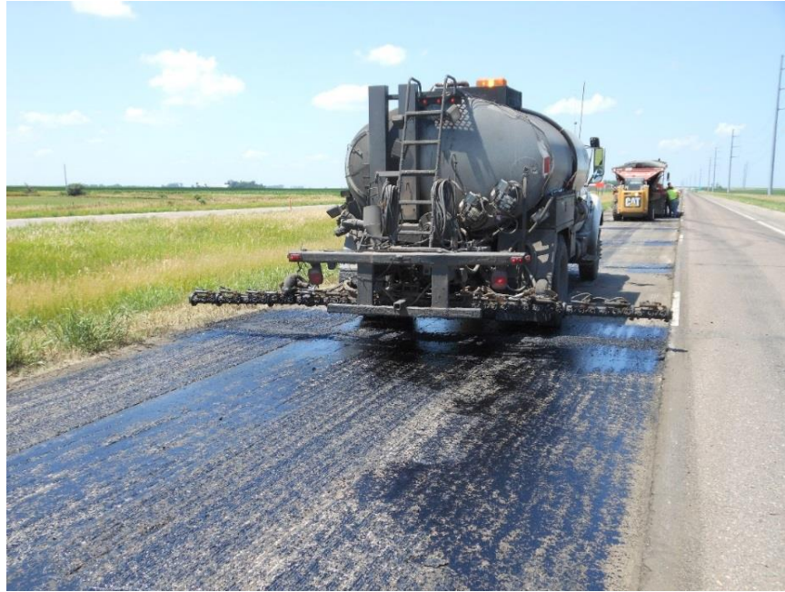
Figure 500.6 – Tack coat distributor truck. Note the streaked appearance. The Contractor should respray this area to achieve uniform coverage.
