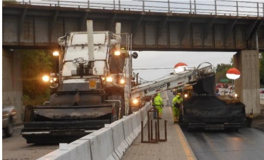
Figure 500.13 – A Material Transfer Vehicle delivers bituminous mixture to the paver. Note that, due to space limitations around the paver, the MTV is in an adjacent lane to the paver. This allows the haul trucks more room to deliver the mix to the MTV.
