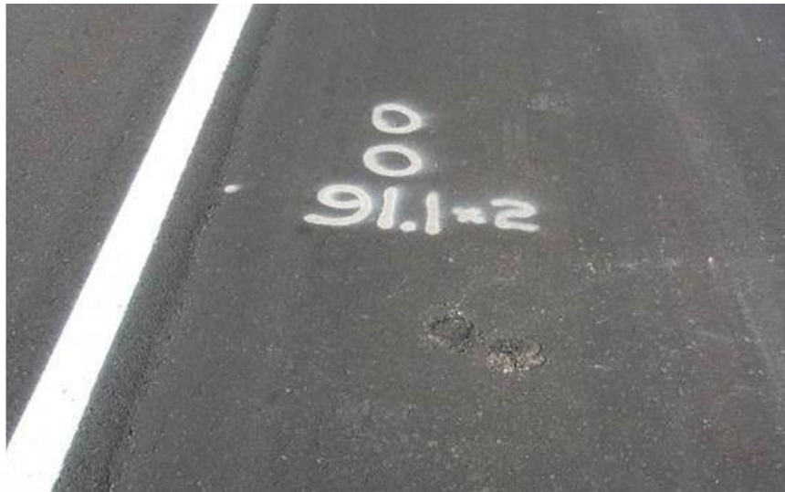
Figure 700.12 – Core locations marked on the roadway. Note that the cores were not taken in the marked locations. These cores must be recored at the proper locations.
