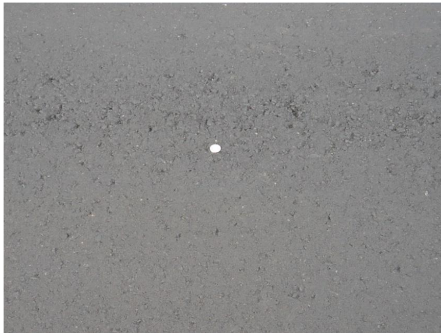
Figure 600.8 – Slightly segregated pavement
