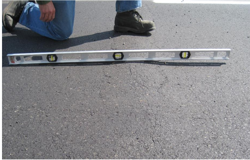
Figure 600.28 – Bump over concrete joint
