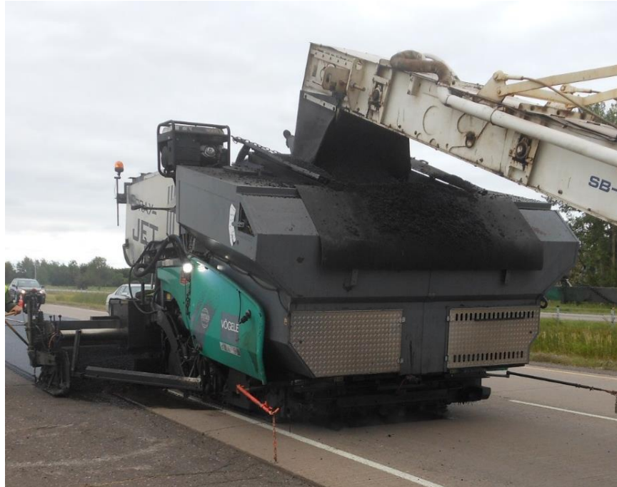
Figure 500.17 – Spray paver in action. Note the tack coat spray bars in front of the screed.
