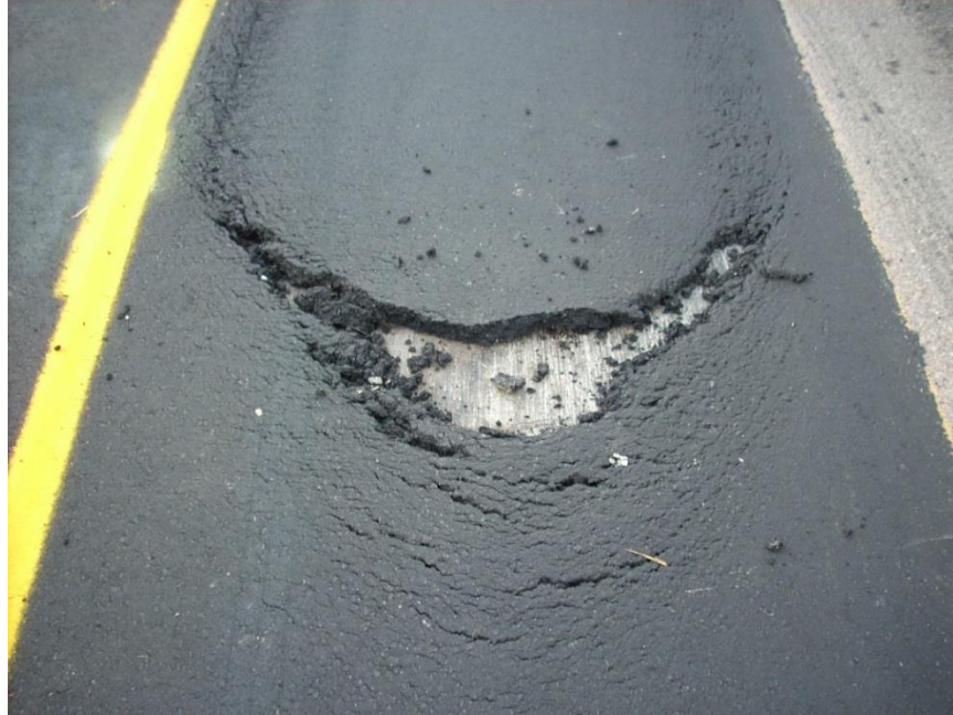
Figure 600.40 – Longitudinal shoving of the bituminous mat as a result of insufficient or nonexistent tack coat. In this case, the wrong bituminous mixture was used for the application in addition to insufficient tack coat prior to paving.
