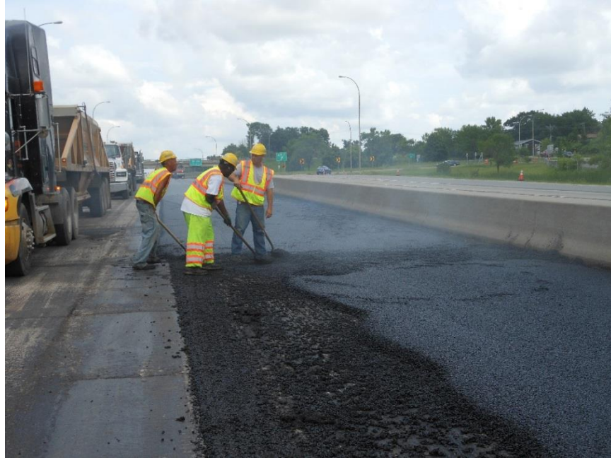
Figure 600.21 – The result of “paving” without bituminous mixture present in the paver hopper
