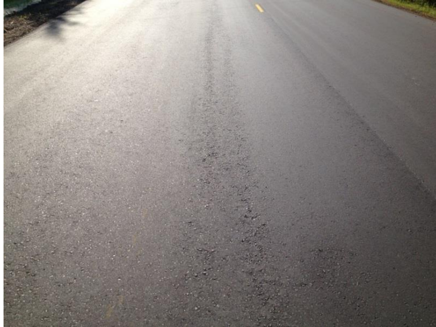
Figure 600.9 – Moderate segregation of the pavement
