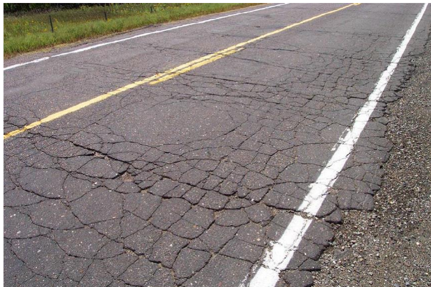
Figure 100.17 – Severe Fatigue Cracking
