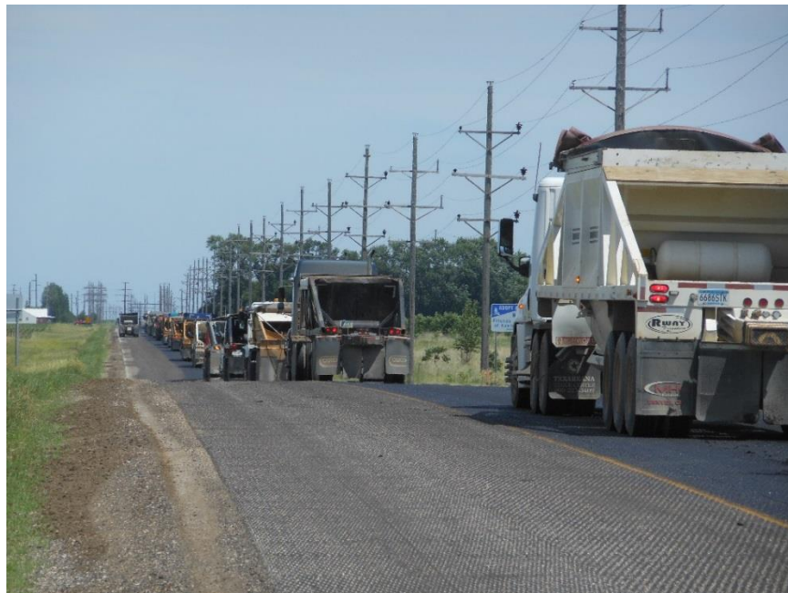
Figure 600.36 – Excessively long truck queue. The bituminous mixture in the truck waiting at the far end of the queue will likely have cooled to an unacceptable temperature.
