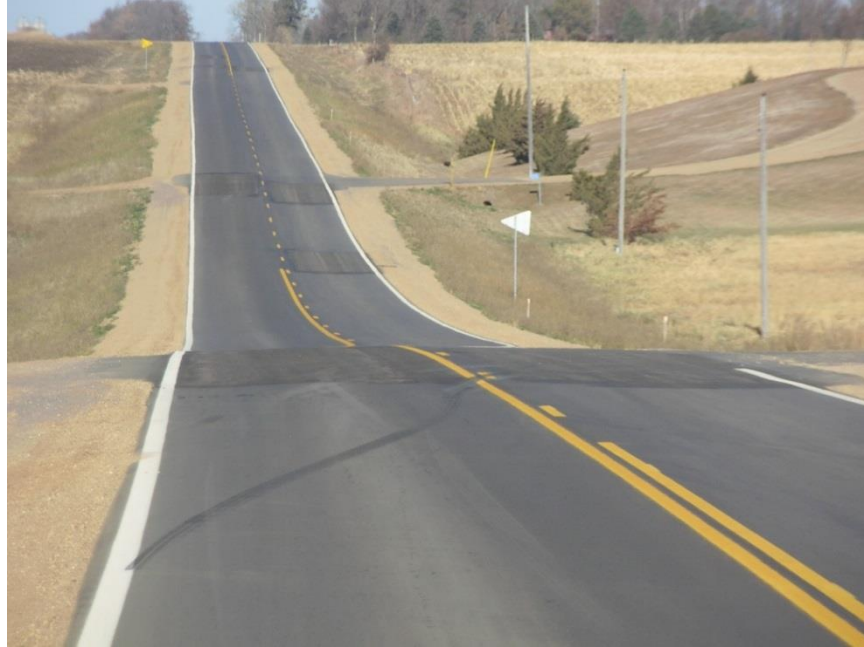
Figure 600.41 – A recently constructed roadway after surface grinding was completed to improve ride quality.
