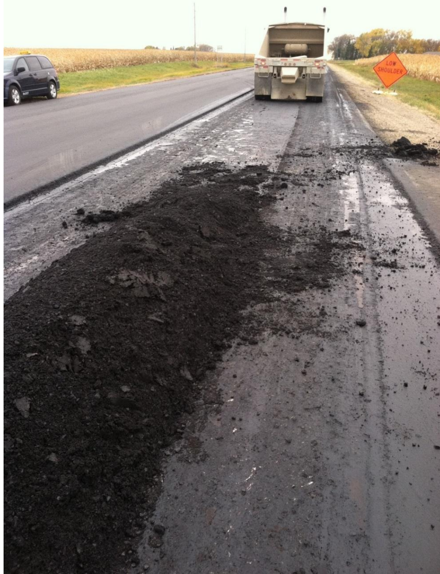
Figure 600.37 – Cold chunks in a windrow. These should be removed.
