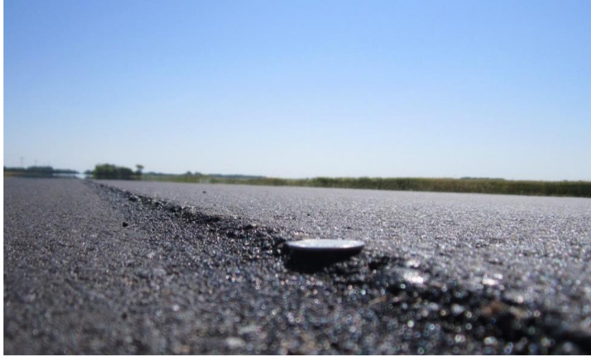
Figure 600.33 – Excessive height differential at a longitudinal joint
