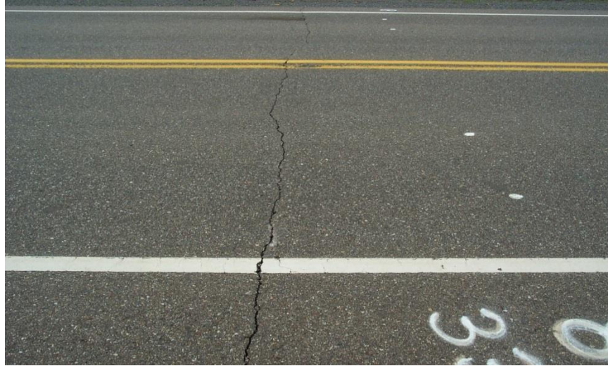
Figure 100.15 – Transverse Thermal Crack
