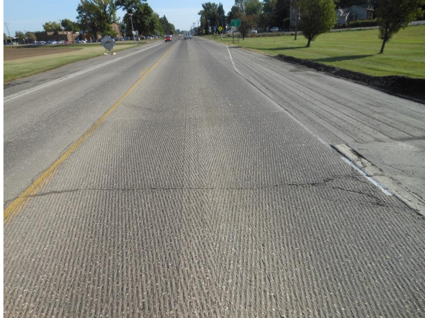
Figure 500.2 – Chevron pattern after milling. Note the angled grooves in the milled surface.
