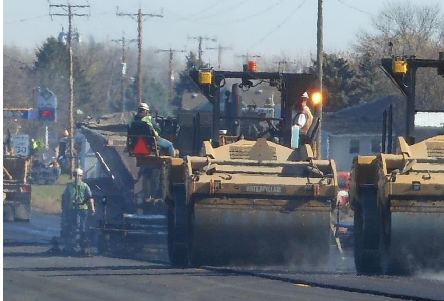
Figure 500.22 – Compacting an unconfined edge. Note the roller at the front of the train hanging the drum over the edge by several inches.
