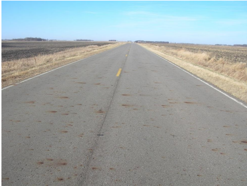
Figure 600.16 – The effect of excessive Iron Oxide in the bituminous mixture.
