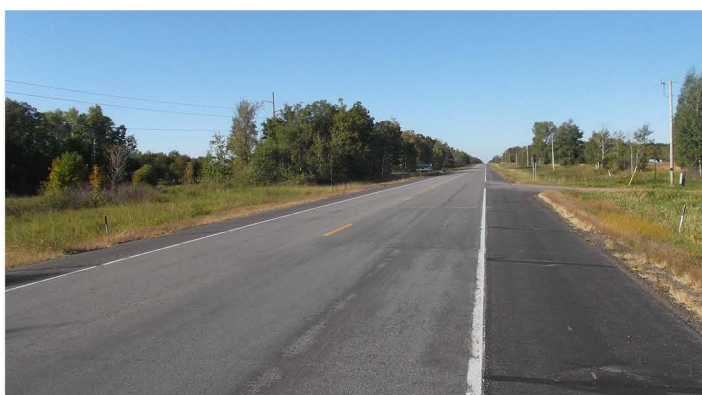
TH 23 Highly Modified Emulsion Right Lane Picture taken 2015. 3 years after placement
