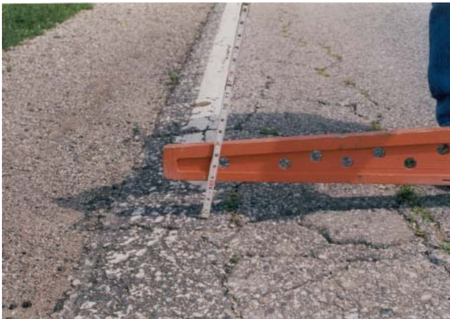
b. Close-up view of pavement damage resulting from edge loading.
