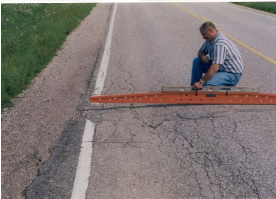
a. Overall pavement damage resulting from edge loading
