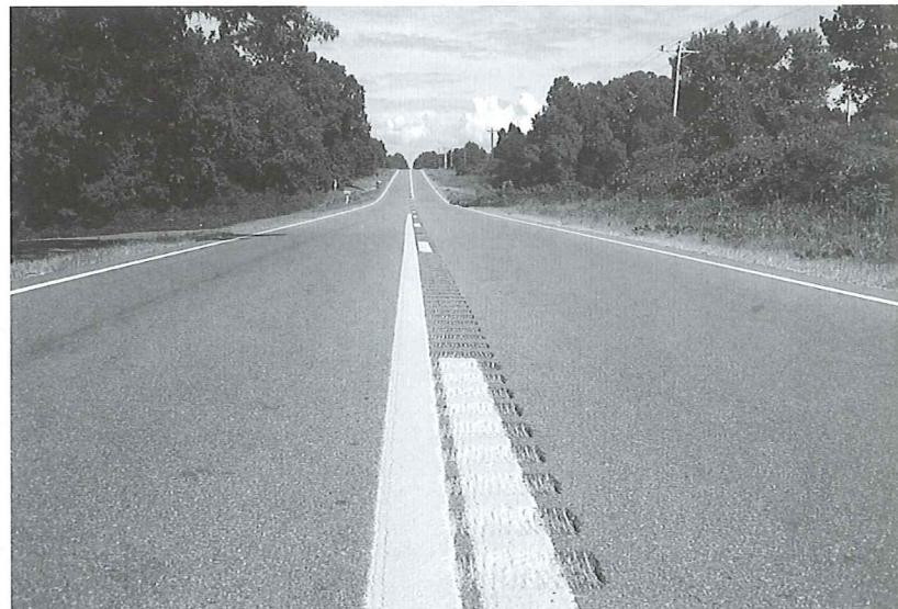
Centerline rumble strips on two lane roads, like this example from Mississippi, can reduce fatalities and injuries from head-on and sideswipe crashes by 44 percent.
