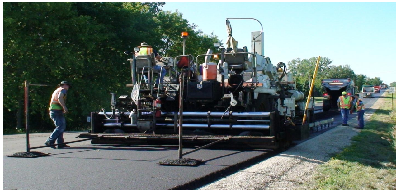
b) – Use of “Ski” During Asphalt Paving to Increase Smoothness of Ride
