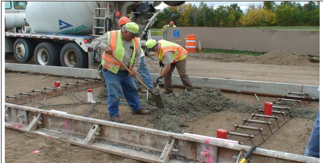
a) – Use of Stainless Steel Dowel Bars in Increase Load Transfer Efficiency
