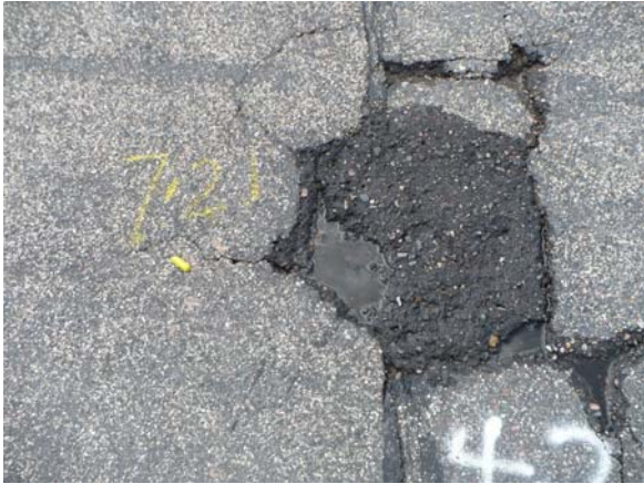
Figure 5 - Condition after 3 months in service 7-21-2009.
