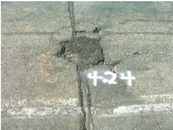
Figure 4 - Condition after 35 days in service 4-24-2009.
