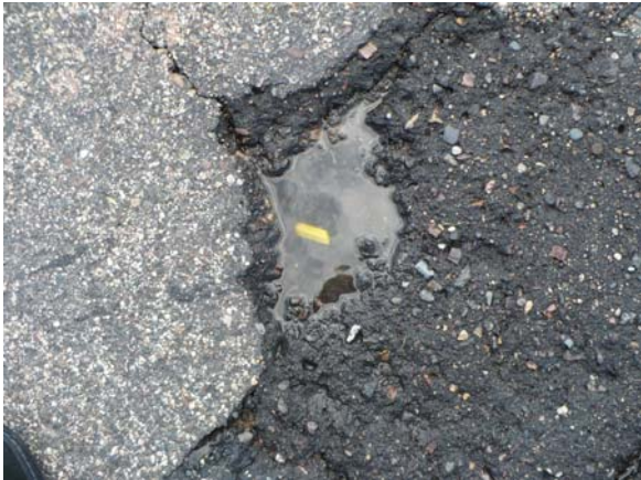
Figure 6 - Condition after 3 months in service 7-21-2009.
