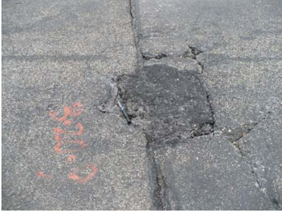
Figure 3 - Condition after 15 days in service 4-4-2009.
