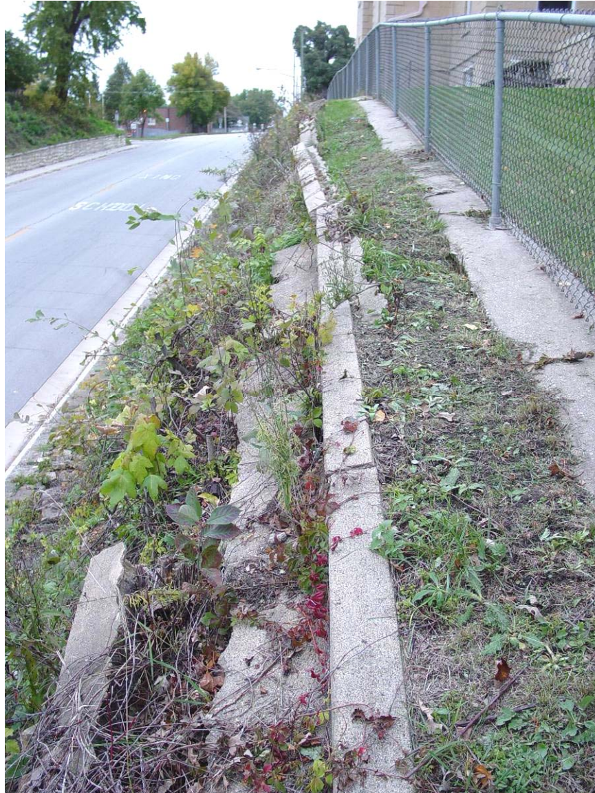
Plate 5. East retaining wall, deteriorated concrete gutter system, facing north
