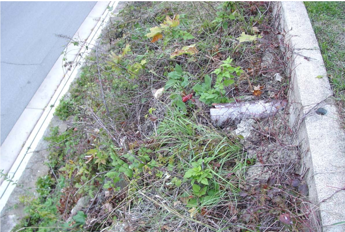
Plate 4. East retaining wall, drainage pipe from Dodge County courthouse downspouts, facing north
