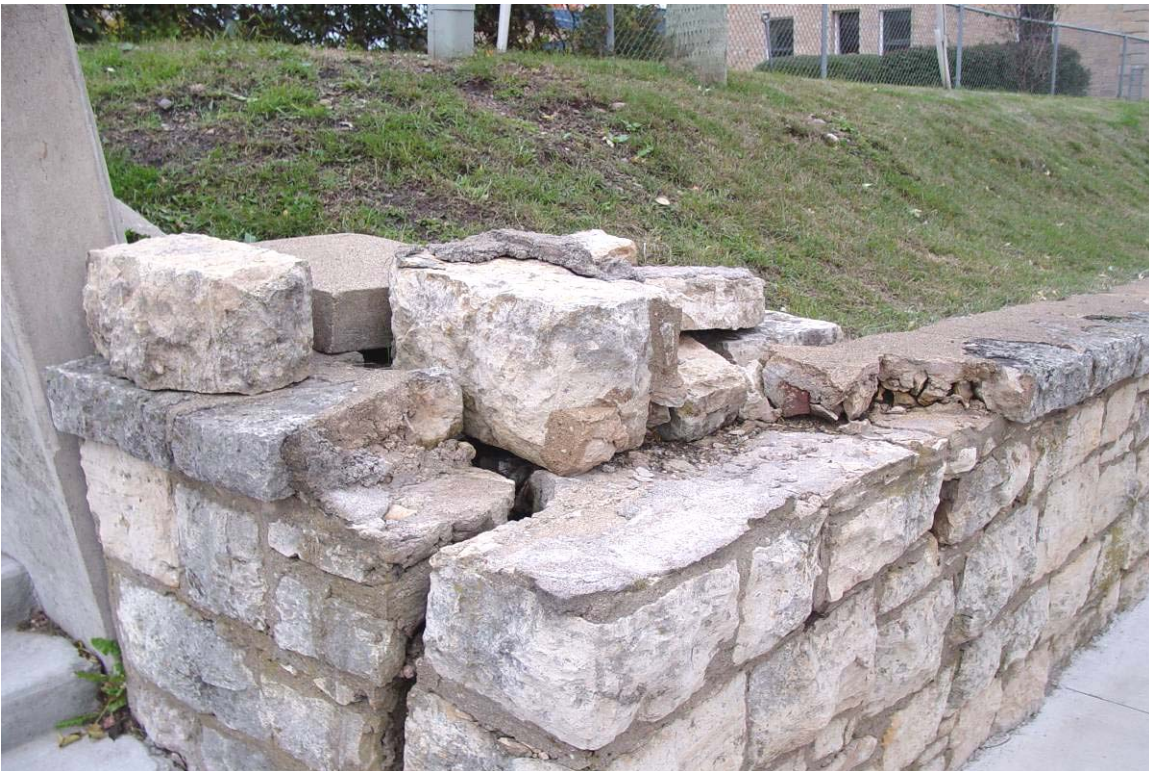
Plate 7. North end of east retaining wall, damaged stone, facing southeast
