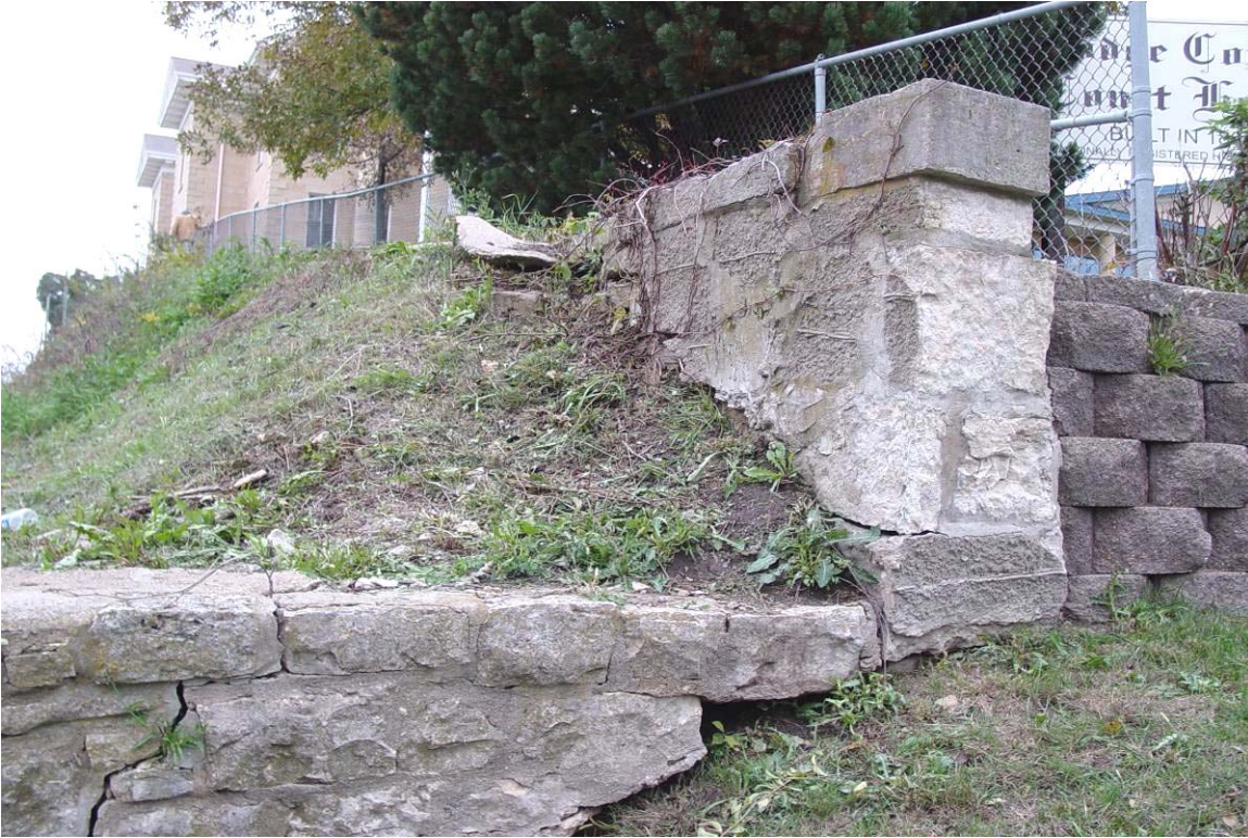
Plate 10. East retaining wall, south end juncture with adjacent retaining walls, facing northeast
