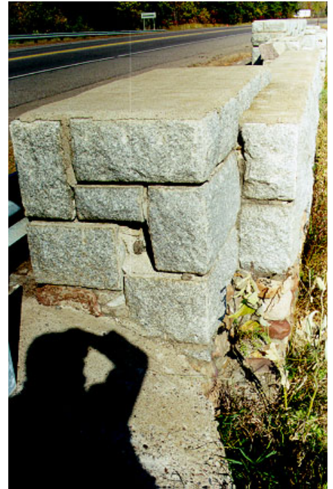
10. Missing Stone and Poor Mortar
