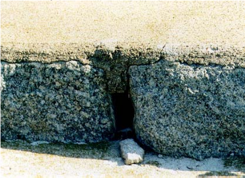
9. Close-up of Mortar Joint Condition.
