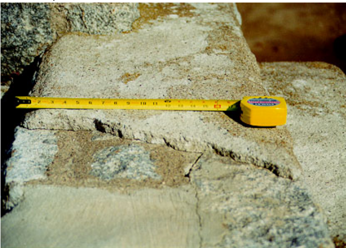
11. Mortar Topping at Walls ( broken and spalling )
