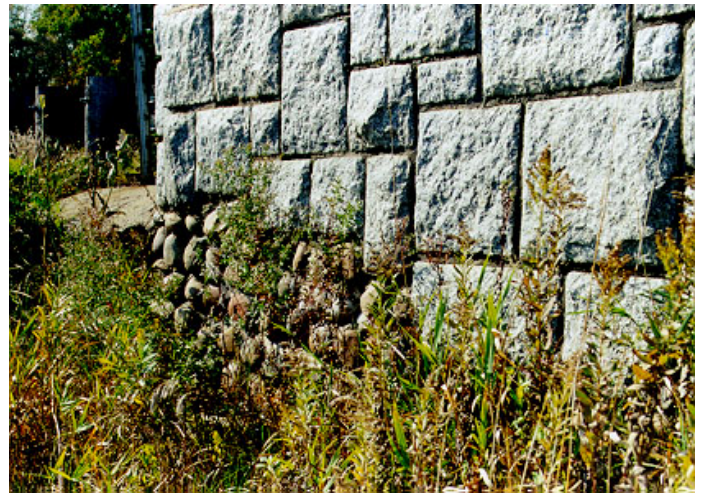
16. Granite/Fieldstone Foundation (Note: fill settling)
