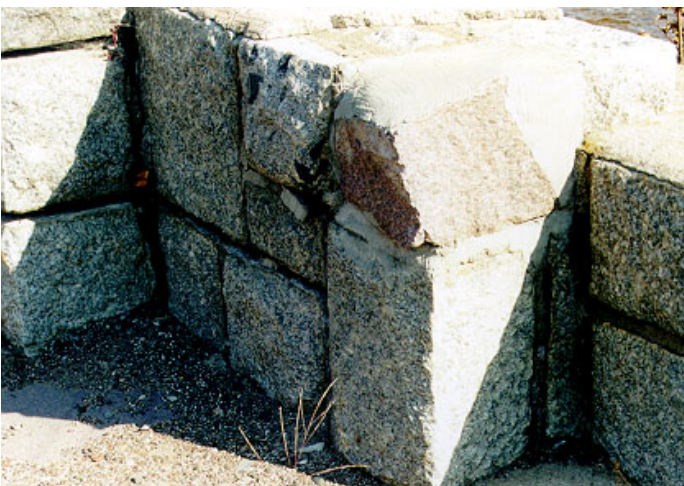
13. Patched End Caps ( spalled mortar topping above sloped stone patch and loose mortar behind )
